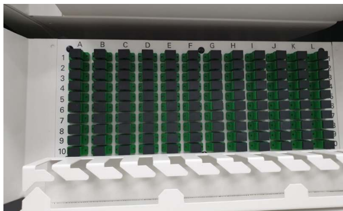
The photo above is an example of the type of ODF deployed at BNL MMR.
